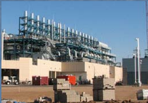
Fab 32 in Arizona. Ramping 45nm in the second half of 2007.
